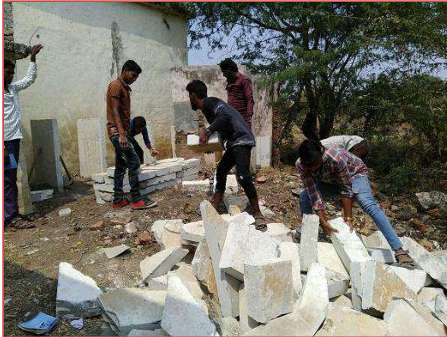
Students constructing toilets for students in Govt. School, Tonasanahalli(s) to Eradicate the open defecation
